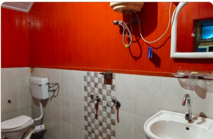
En-Suite Bathroom with Hot Water Geyser
